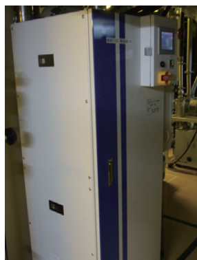
VOC treatment equipment
